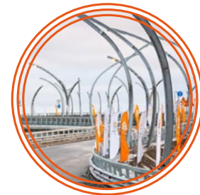
Construction of the Western High-Speed Diameter interchange in the Shkipersky Protok area
