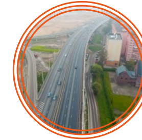
Construction of exits from the bridge crossing over the Staraya and Novaya Pregolya rivers and a transport interchange in the area of Solnechny Boulevard in Kaliningrad
