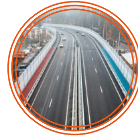
Construction of a transport interchange in the Vsevolozhsk district. The facility was included in the TOP 5 of the national project "Safe Quality Roads"
