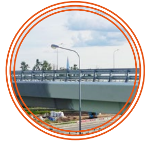
Construction of an adjoining road to the Ring Road interchange to the "Airport complex at the Levashovo airfield" facility
